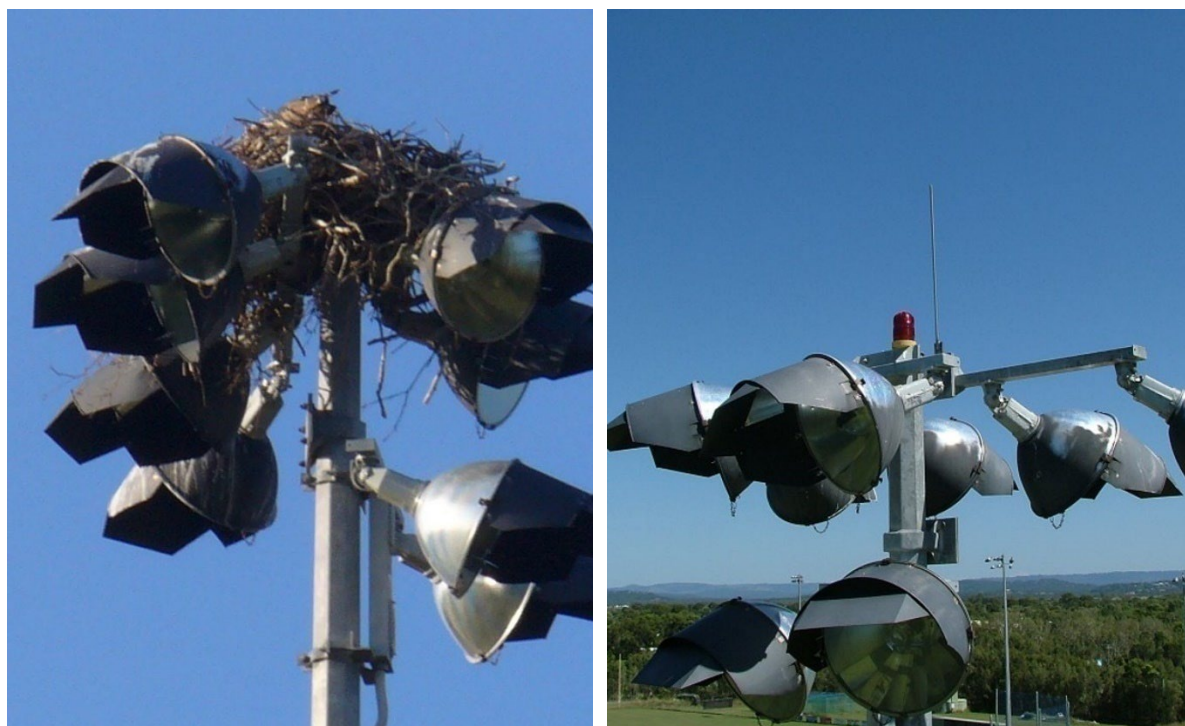
Figure 12 Bird nest (left) and non-harmful spike as a nesting deterrent following removal (right) (Source Avisure)
